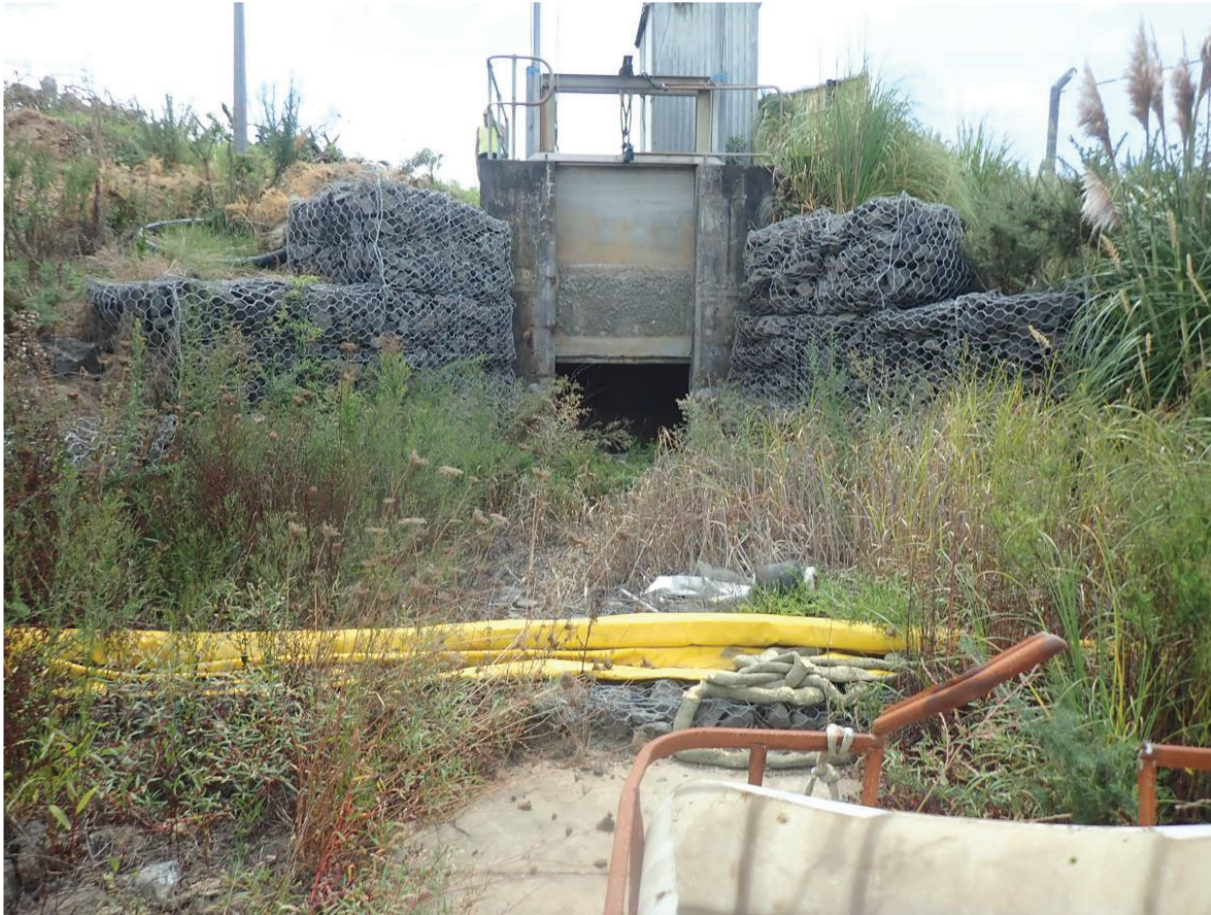
Figure 11: Floodgate at the water-cooling pond outlet
