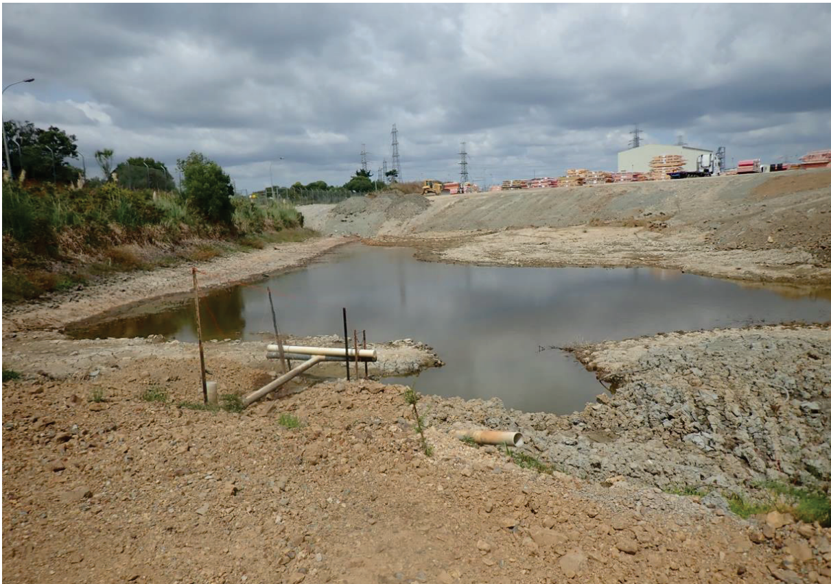
Figure 4: Remainder of the water cooling pond being used as a sediment control pond
