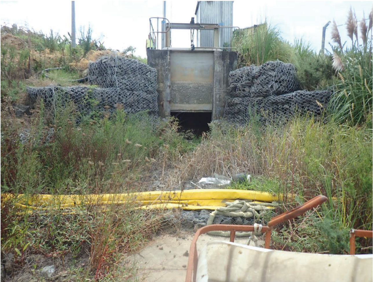
Figure 11: Floodgate at the water-cooling pond outlet
