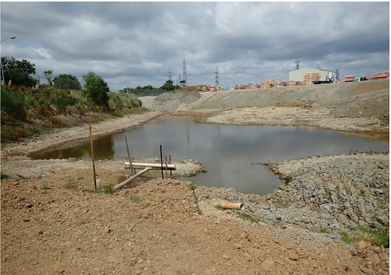
Figure 4: Remainder of the water cooling pond being used as a sediment control pond
